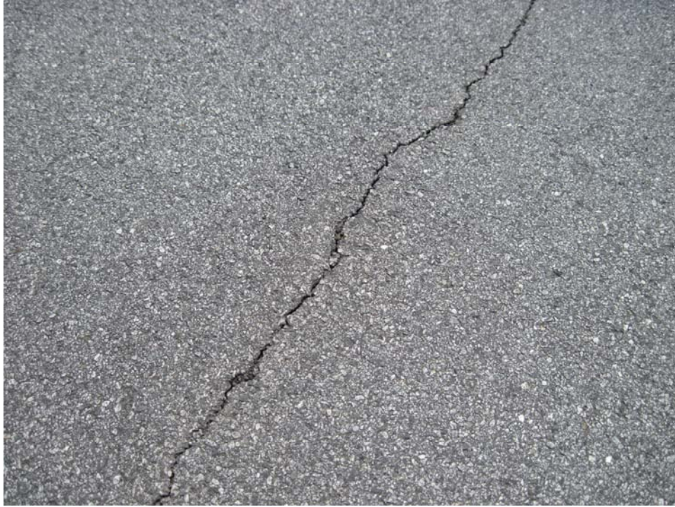
R2L20RAP-20. Longitudinal and Transverse Cracking (Sample Unit #02).
