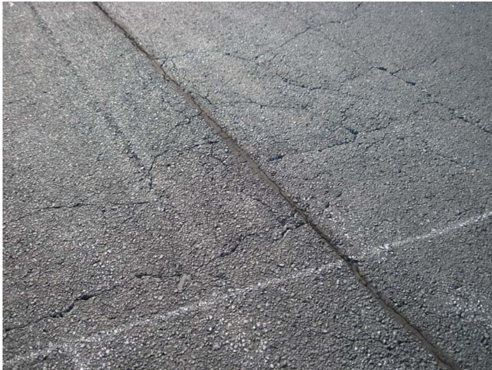
R927AP-10. Alligator Cracking (Sample Unit #51).
