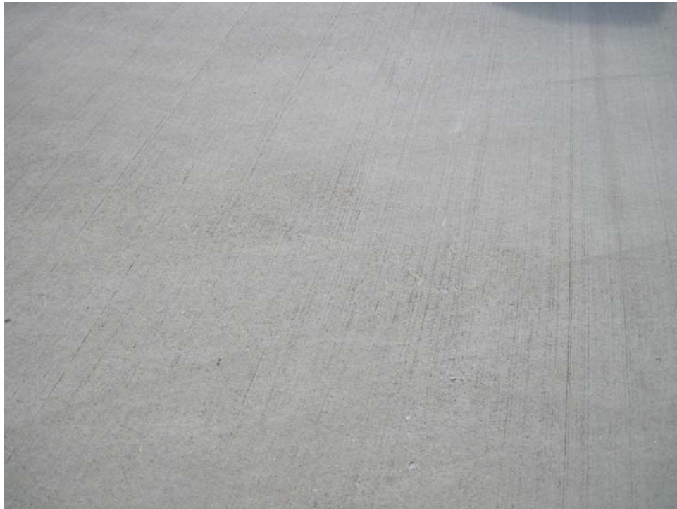
TARUNUPAP-10. Shrinkage Cracking (Sample Unit #02).
