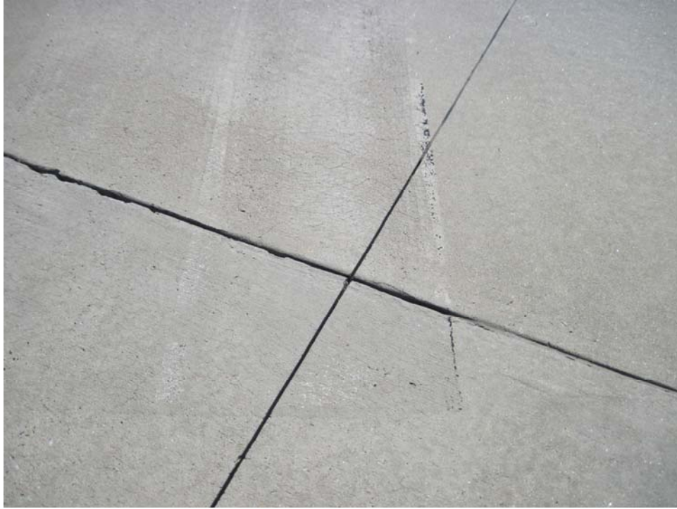
TAAP-20. Joint Seal Damage (Sample Unit #02).
