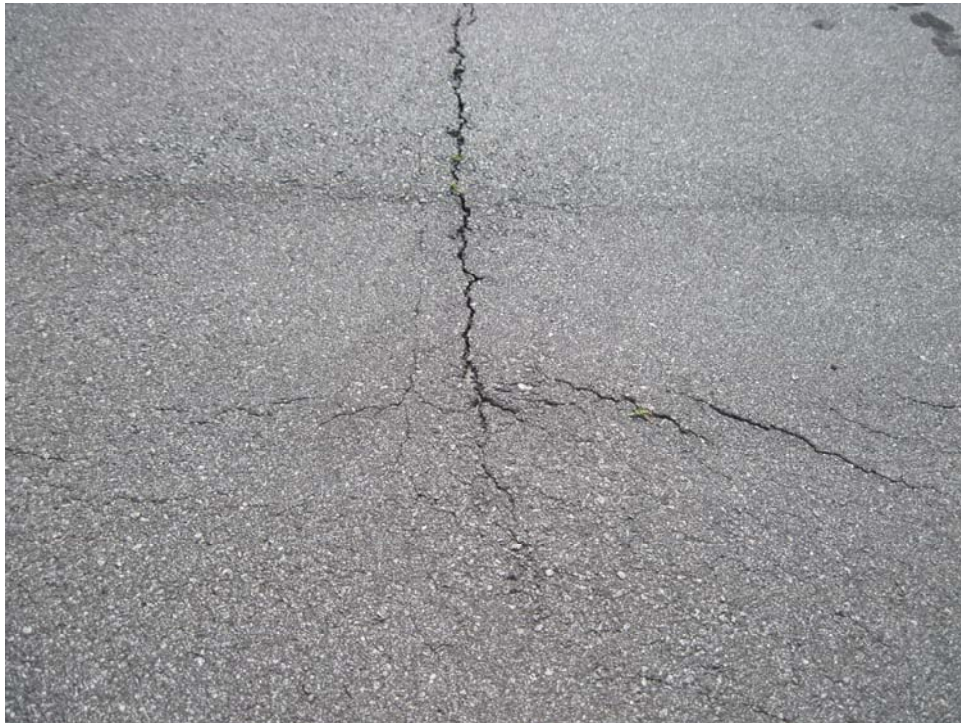
APERIMAP-30. Longitudinal and Transverse Cracking.
