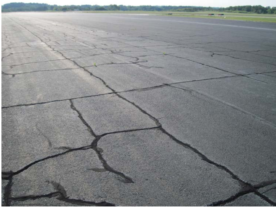
R927AP-10. Block Cracking (Sample Unit #64).
