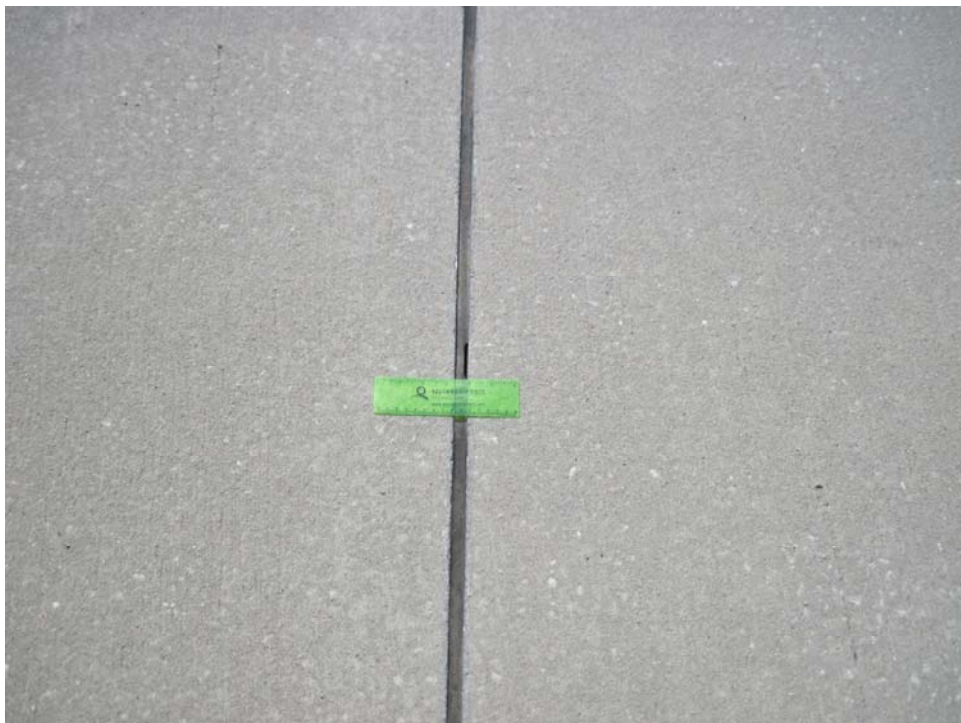
THAP-10. Joint Seal Damage (Sample Unit #02).
