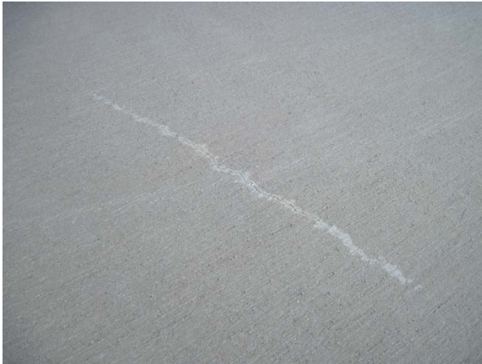
TEAP-10. Shrinkage Cracking.
