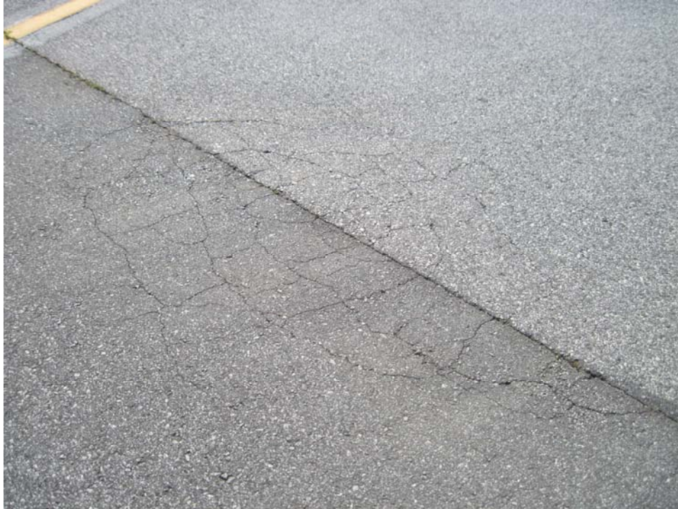
TDAP-30. Alligator Cracking (Sample Unit #03).
