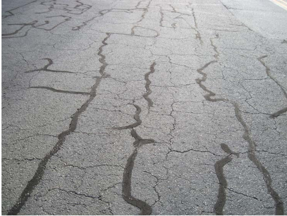
APERIMAP-10. Alligator Cracking (Sample Unit #05).
