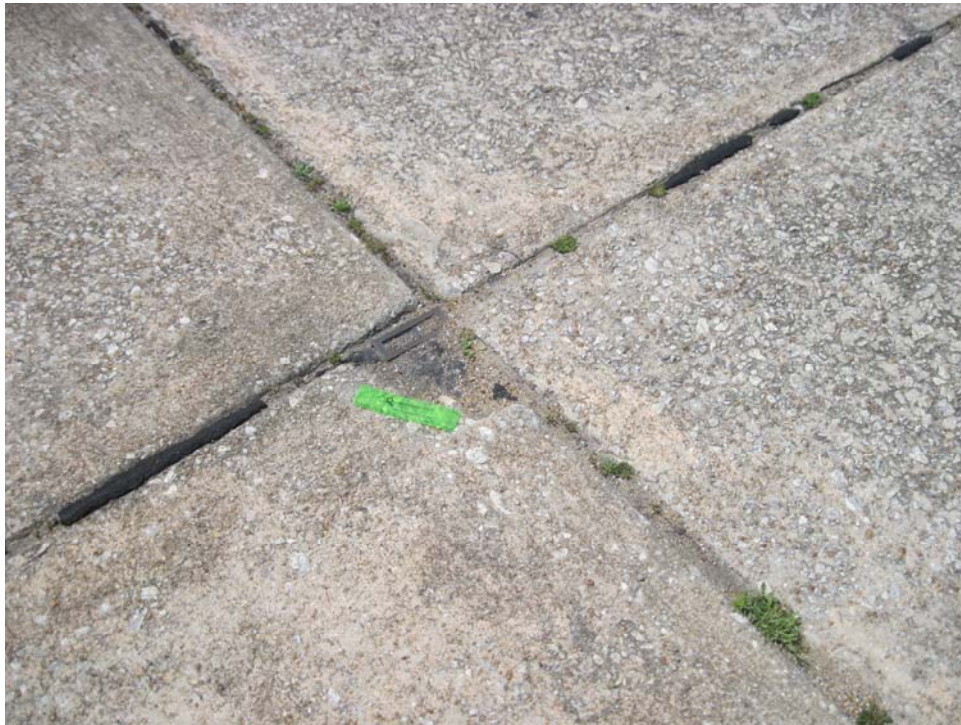
ANWRAMPAP-20. Corner Spalling (Sample Unit #22).
