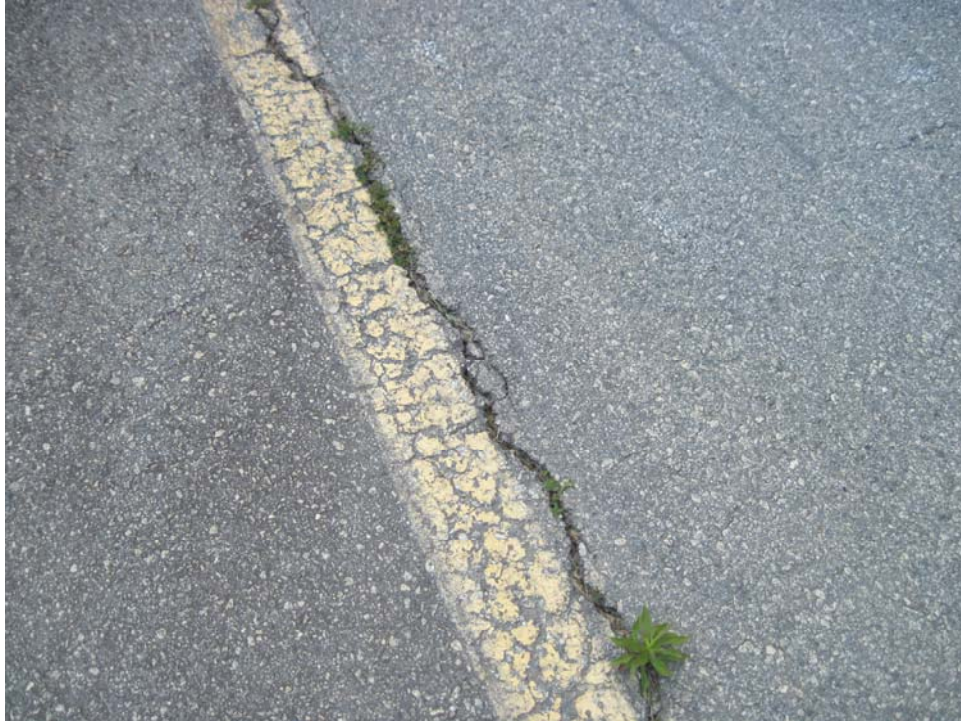
HELIAP-10. Unsatisfactory Paint.
