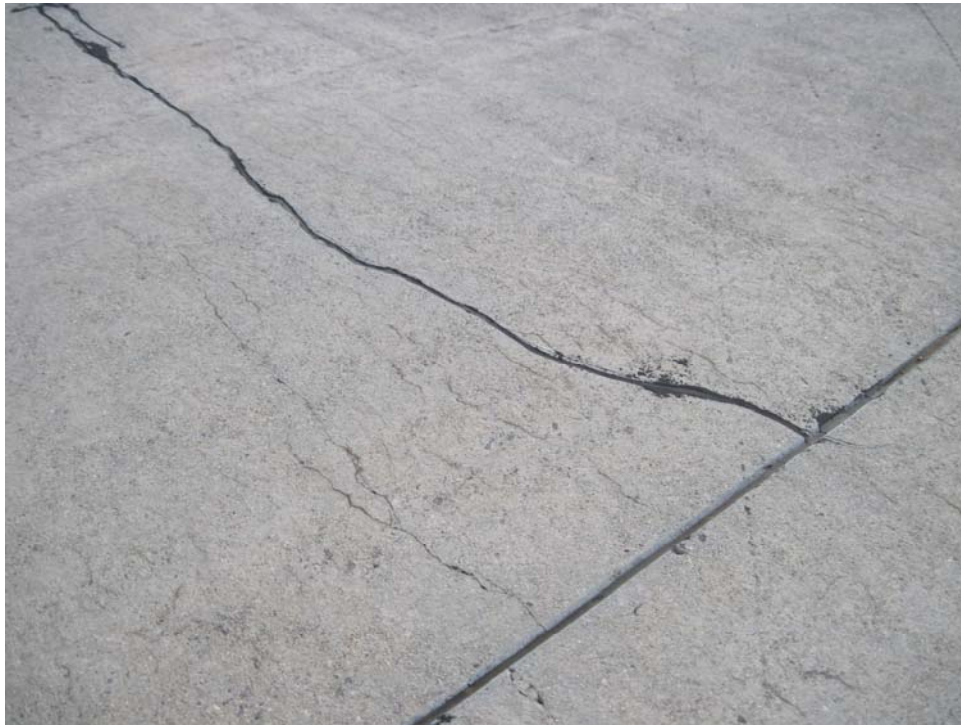
TAAP-30. LTD Cracking and ASR (Sample Unit #04) (1).
