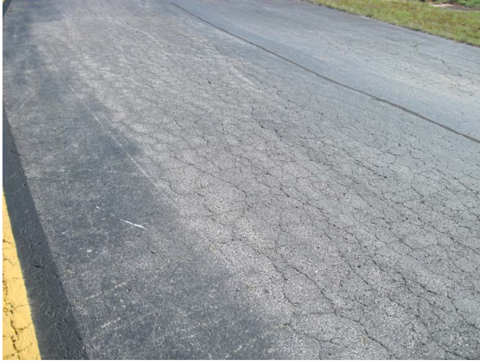
TDAP-10. Alligator Cracking (Sample Unit #16).
