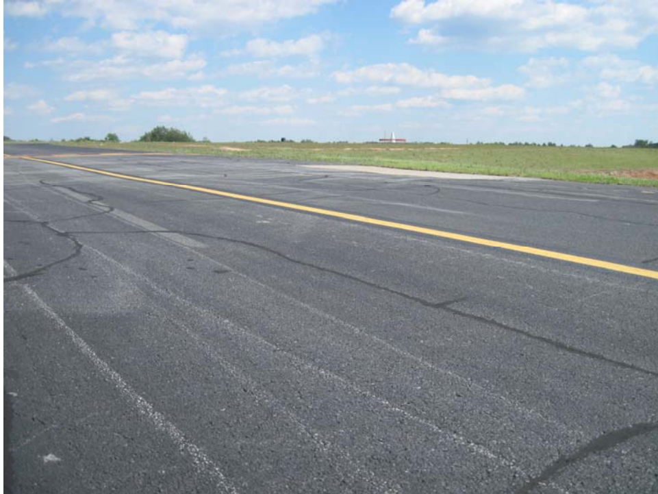
TGAP-10. Rutting (Sample Unit #04).
