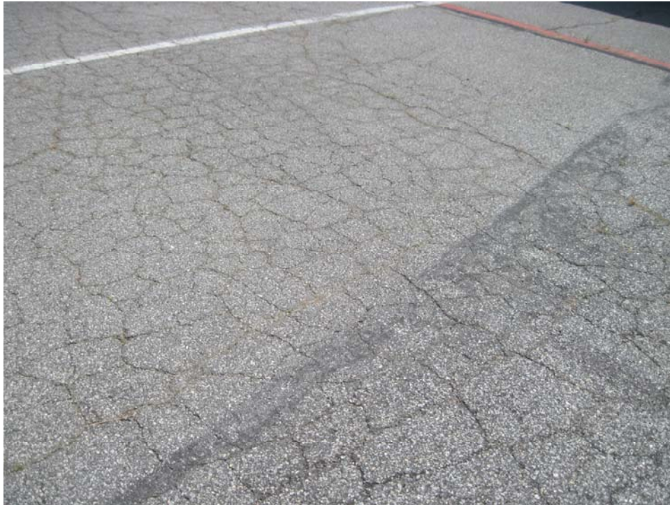
ANRAMPAP-10. Alligator Cracking (Sample Unit #64).
