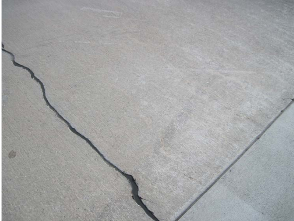
TAAP-30. LTD Cracking and ASR (Sample Unit #29) (2).
