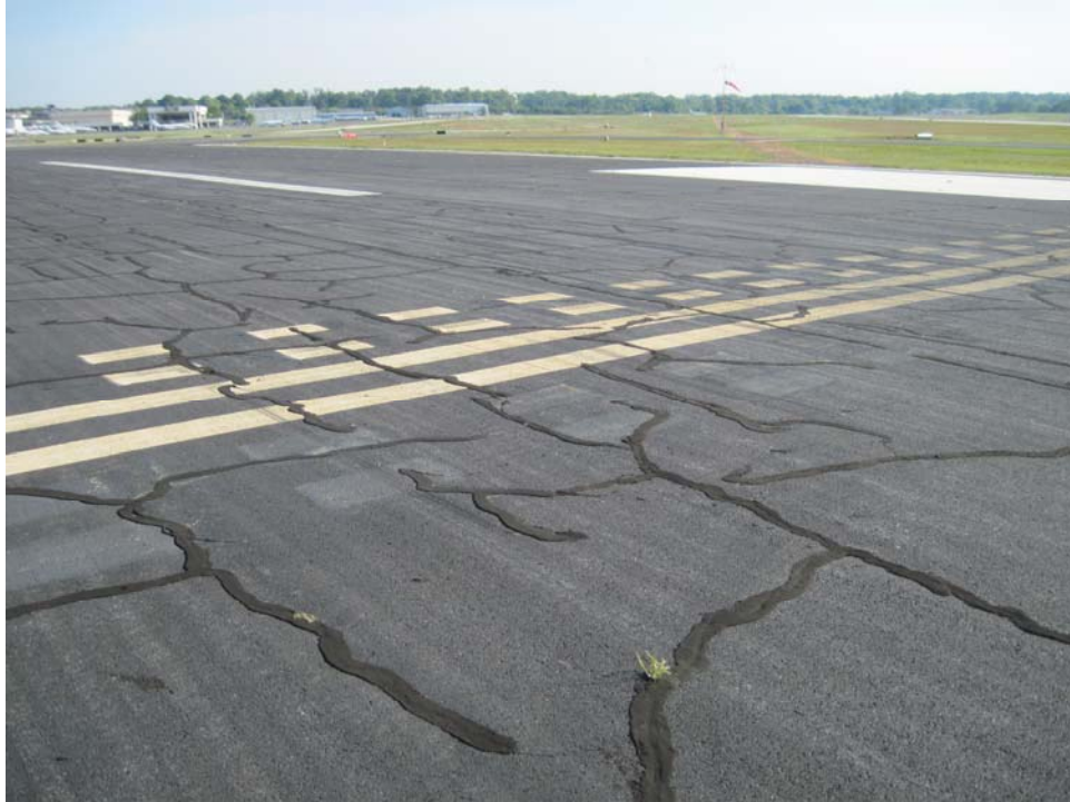
R1634AP-10. Block Cracking (Sample Unit #42).
