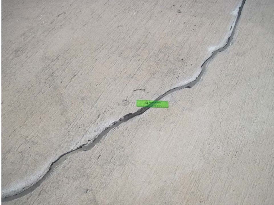
TAAP-10. LTD Cracking (Sample Unit #12).
