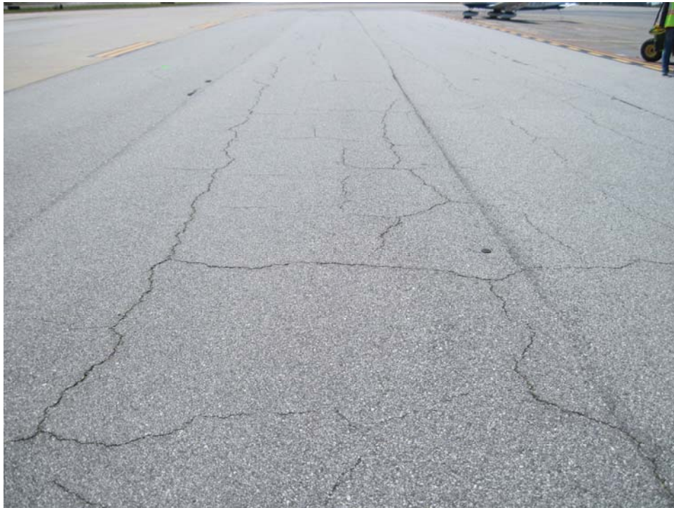
APERIMAP-20. Block Cracking (Sample Unit #05).
