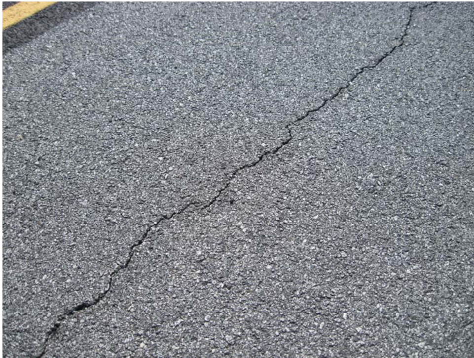
TDAP-20. Longitudinal and Transverse Cracking and Weathering (Sample Unit #06).
