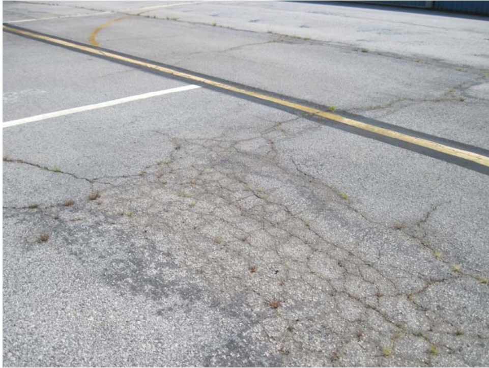
ANERAMPAP-10. Alligator Cracking.
