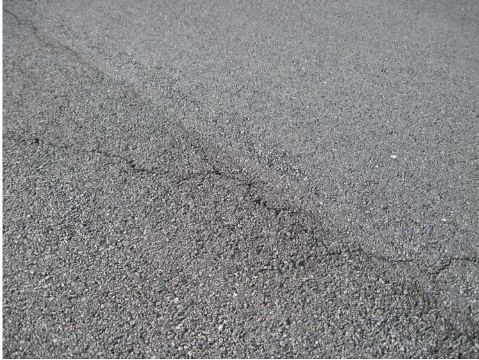
TFAP-10. Longitudinal and Transverse Cracking and Weathering (Sample Unit #04).
