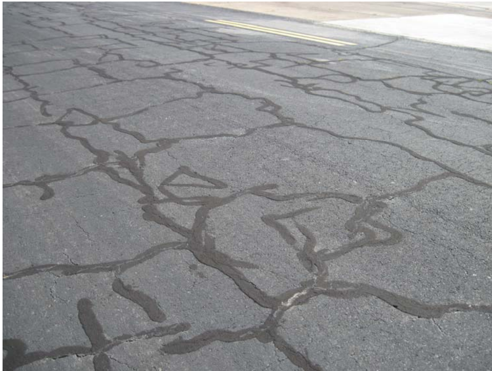
TBAP-10. Block Cracking (Sample Unit #04).
