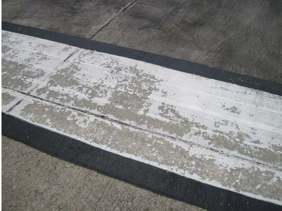
HELIAP-20. Unsatisfactory Paint.
