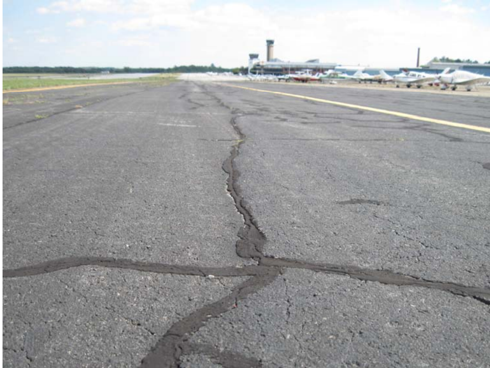
TBAP-10. Rutting (Sample Unit #03).
