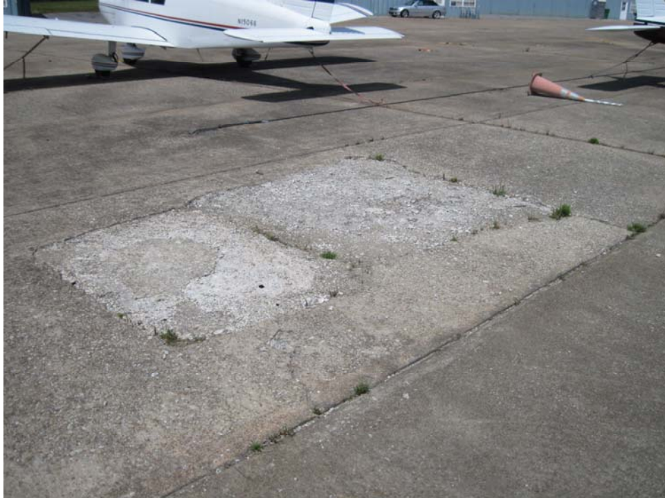
ANWRAMPAP-20. Shattered Slab and Scaling (Sample Unit #22).
