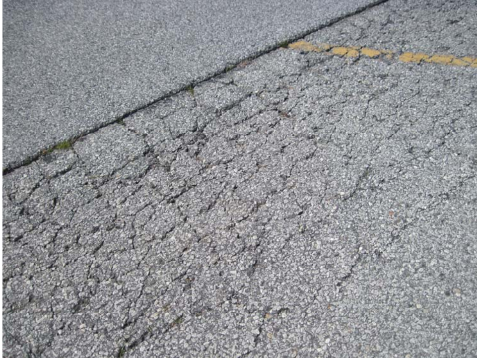
TKAP-20. Alligator Cracking and Rutting (Sample Unit #19).
