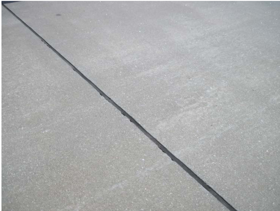
TBAP-20. Joint Seal Damage (Sample Unit #16).
