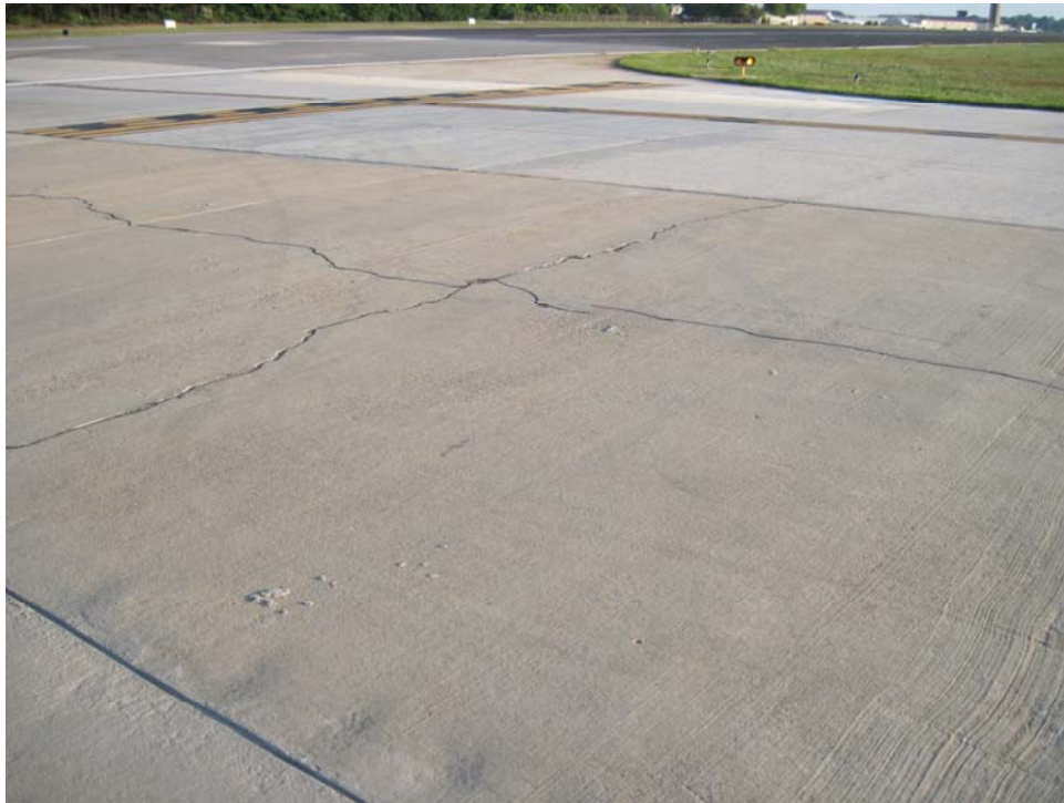
TAAP-10. Shattered Slab (Sample Unit #04).
