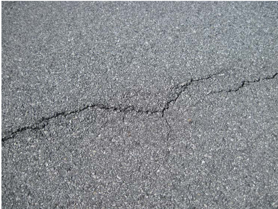
TCAP-10. Longitudinal and Transverse Cracking and Weathering (Sample Unit #02).
