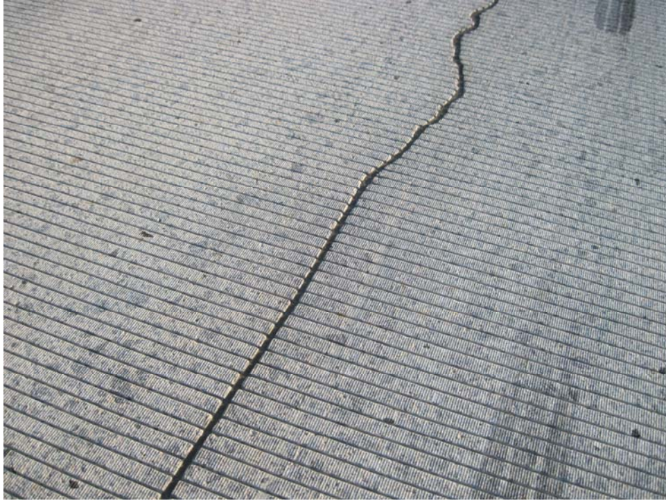
R2R20LAP-10. LTD Cracking (Sample Unit #12).
