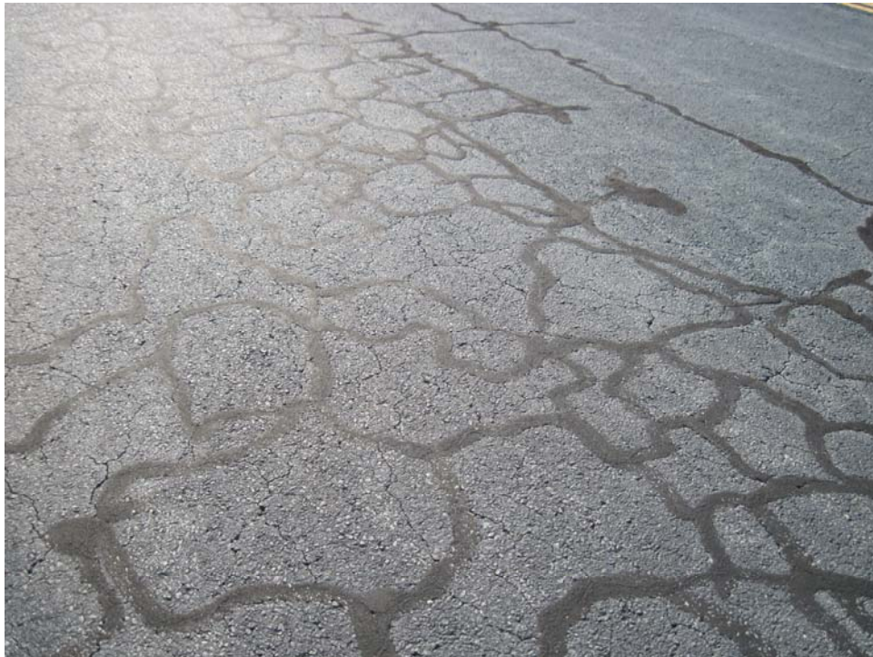
TCAP-30. Alligator Cracking (Sample Unit #01).
