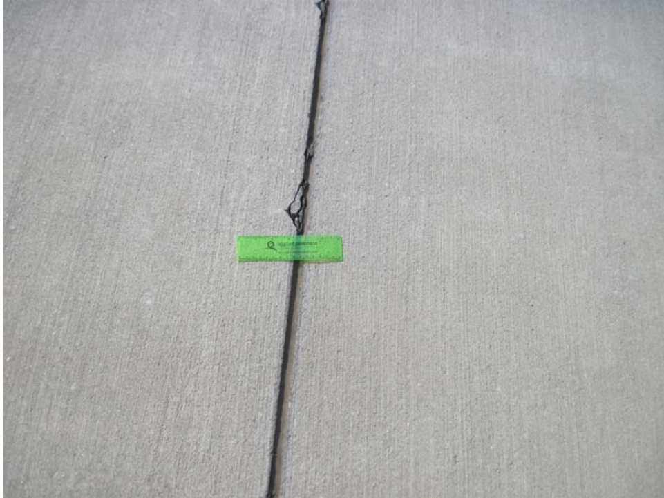
TEAP-20. Joint Seal Damage (Sample Unit #07).
