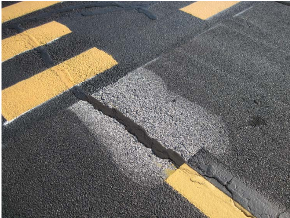
TBAP-40. Weathering and Longitudinal and Transverse Cracking (Sample Unit #4).
