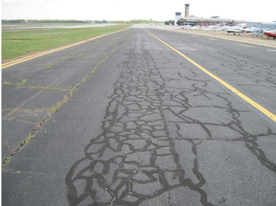
TBAP-10. Alligator Cracking (Sample Unit #07).
